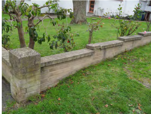
Picture 4.29 Low wall to one front garden along Lower Kerry Avenue - these are characteristic of the area and emphasise the impact of the softly landscaped front gardens
