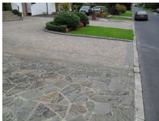
Picture 4.108 Excessive hardsurfacing introduces a barren appearance at odds with the intended design of the Conservation Area
