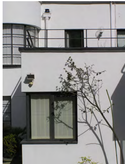
Picture 4.63 Flat roof with sundeck feature on number 6 Kerry Avenue, key to its Modernist Design
