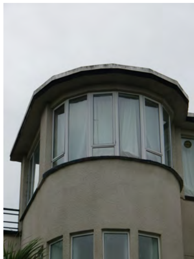
Picture 4.84 Replacement of original Crittall windows here detracts from the intended delicate nature of these windows and the strong geometrical lines and form of the buildings
