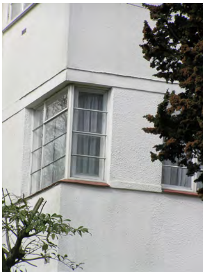
Picture 4.78 Crittall windows sometimes follow the sharp corner of a building to emphasise the strong geometrical forms as above, and in the picture right, on number 2 Valencia Road
